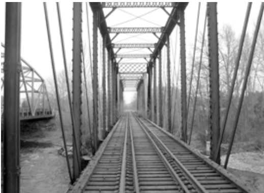
The Rail banked section from 40th ave. out to Naches includes this bridge crossing on the Naches River just east of Glead, next to Highway 12, will be used to create a connection for the Yakima Greenway to our neighbors in Glead and Naches.
